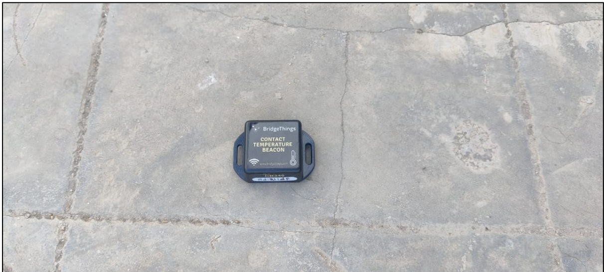
Figure 11 Surface Temperature Logger Placed in Ladies Hostel 2 Roof
