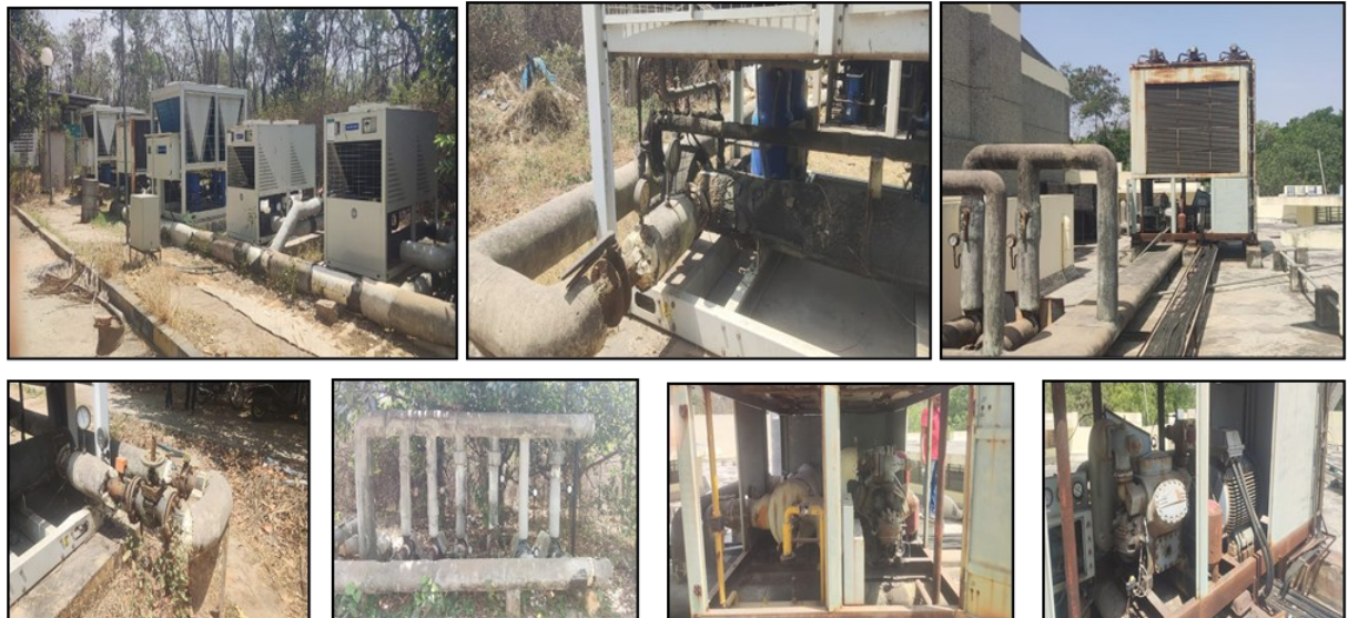
Figure 2 Condition of Existing Chiller Systems
