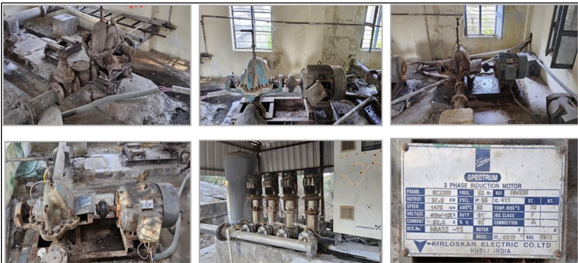
Figure 6 Current Condition of Motors & Pumps in the Main Pump House
